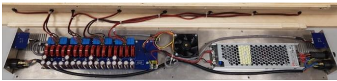
Figure 3 – Interiors of the electronics compartment.
