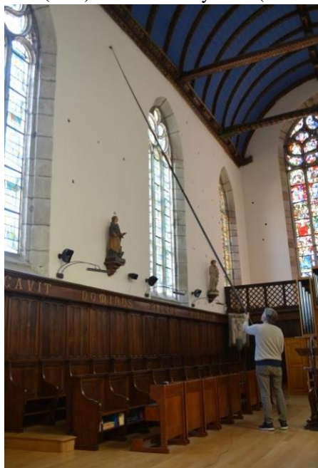
Figure 1 – West wall of the liturgical choir of the Abbey “Couvent des Ursulines” formerly “Saint-François de Cuburien”, Saint-Martin des Champs (close to Morlaix), 16 th century (Photo credit: B. Bertholon)
